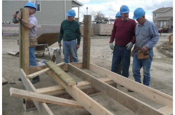
Four men (hard at work???) on the construction of part of a house
